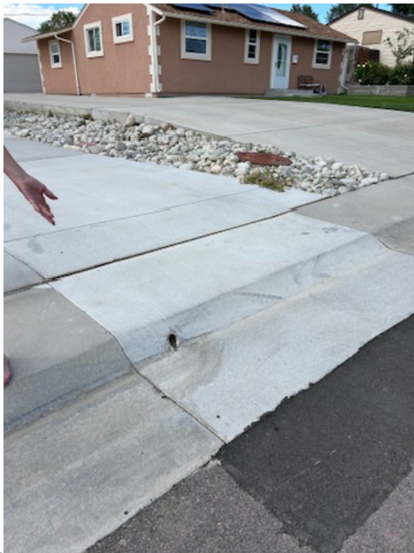
Figure 7 – Campo St June 2026 - The "water feature" on Campo. Water pours out from under the sidewalk during heavy rains. Questioning how the Reservoir was decommissioned.
