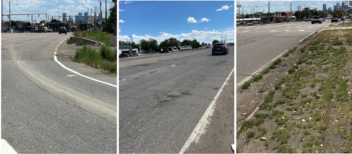
Figure 8 Road conditions and lack of sidewalk on south bound Broadway just beyond the Highway 36 off ramp. July 30, 2026
