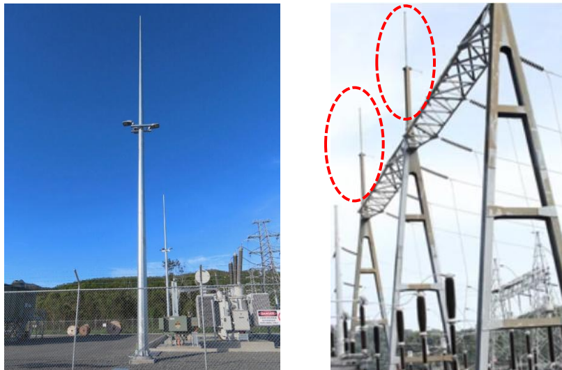
Pictured: Standalone lightning protection mast (left) and lightning masts affixed to substation/transmission infrastructure (right)
